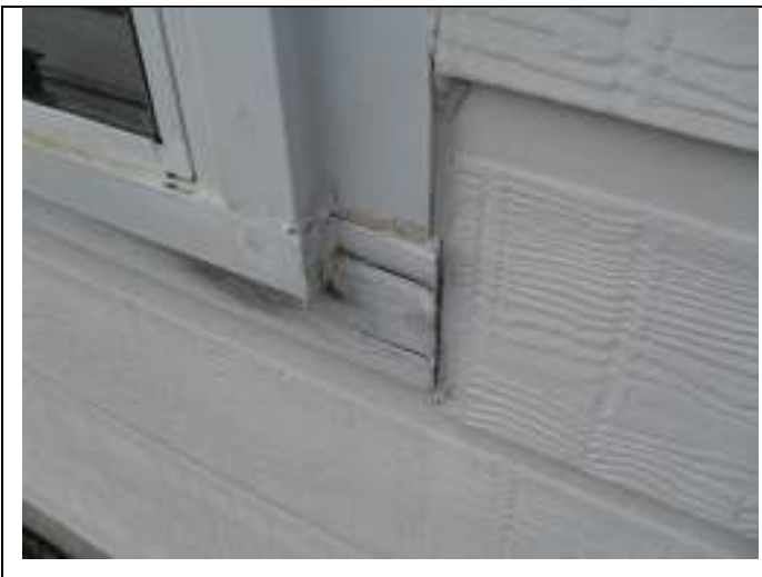
Sample of wood rot of rear exterior trim
