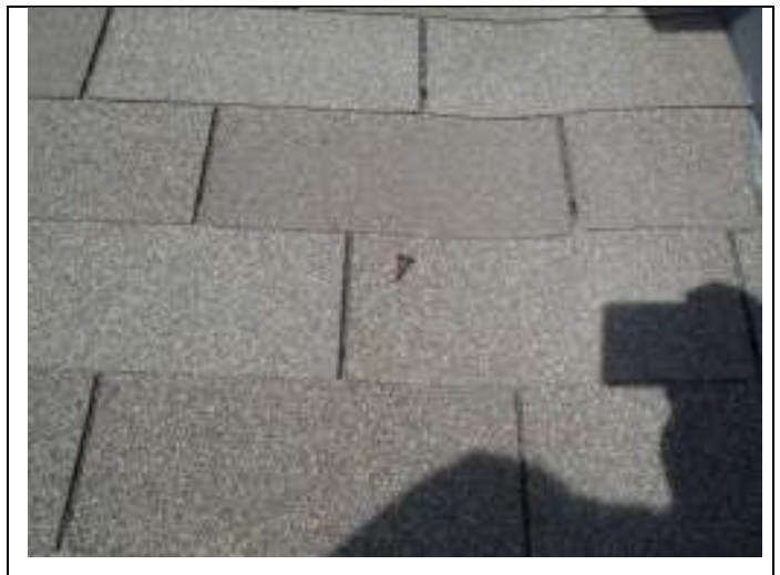
Sample of exposed nail in the roof
