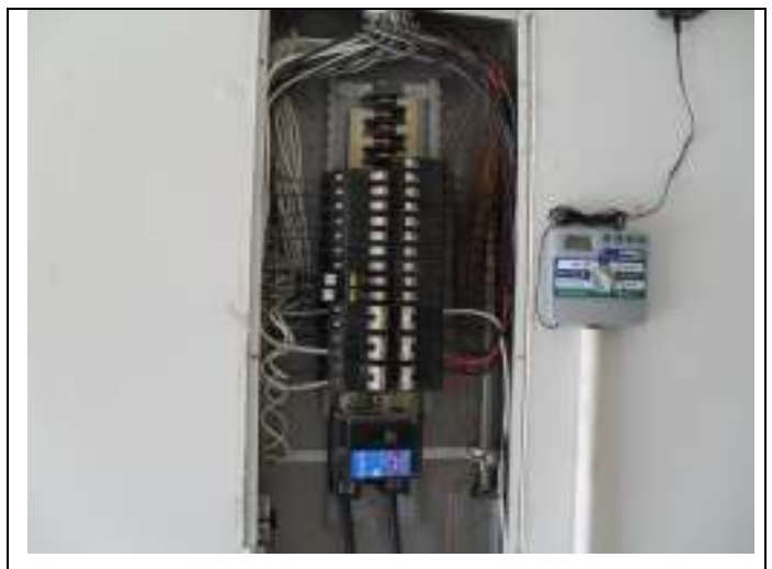
Photo of main electrical panel with cover removed
